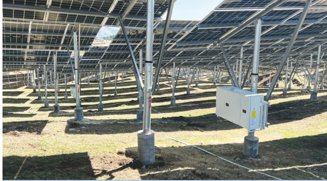
China Yunnan Qiaojia Project 240MW
