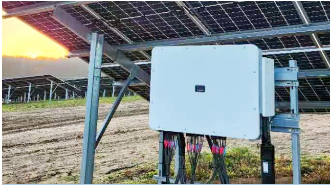
Romania Photovoltaic Project 54MW
