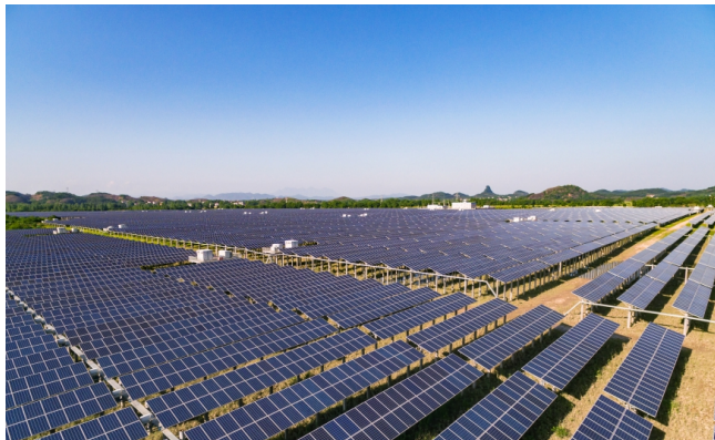
China Bayannaoer Project 800MW
