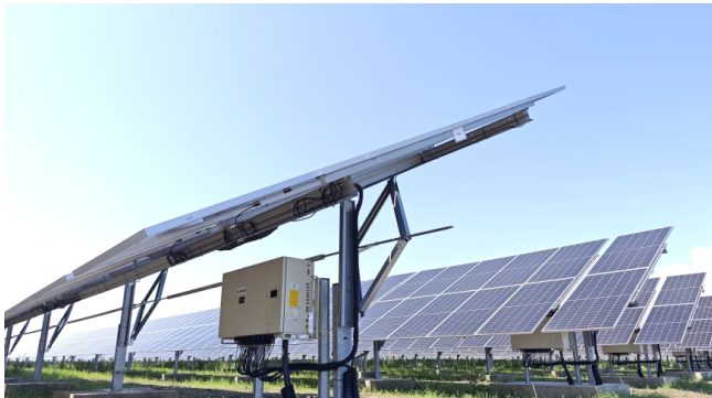
Spain Ohla Project 230MW
