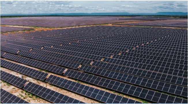
Brazil Ufv Marangatu Project 446MW
