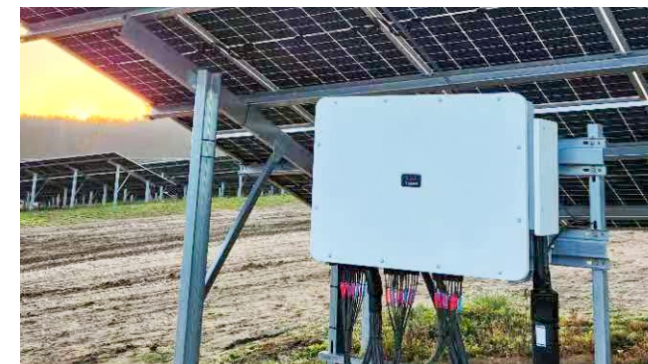
Romania Photovoltaic Project 54MW
