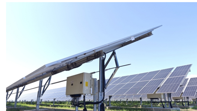
Spain Ohla Project 230MW
